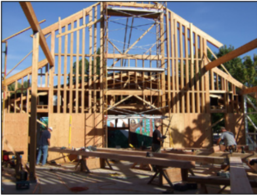
Malakai Schindel's mural of St. Francis and native Mendocino County wildlife on the side of the present church building can be glimpsed through the new construction in Willits, California (Photo by Bill Bruneau)
